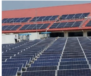
Chandon India: photovoltaic panels to cool wine cellars.
