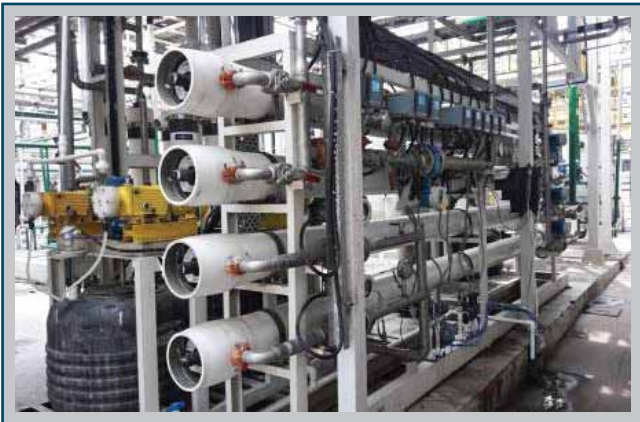
Tertiary RO unit installed at Manesar
