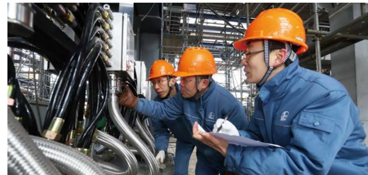
Qilu Petrochemical staff inspect the refrigeration unit of the CCUS project
