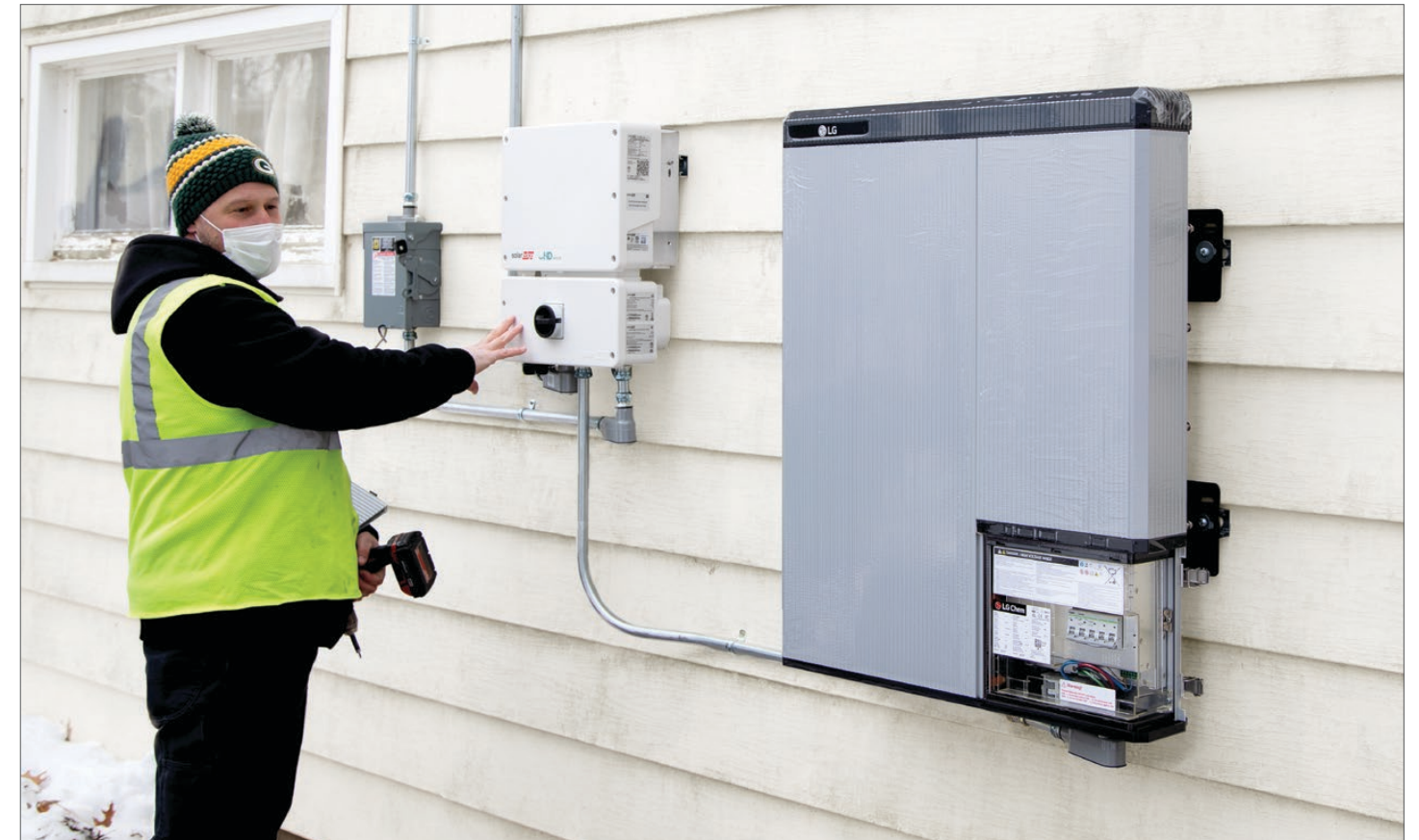
MGE is partnering with a number of homeowners who have rooftop solar arrays to test residential battery storage to better understand how the technology could be used to manage peak demand and to enhance reliability.
