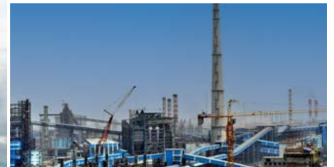
RINL- Coke and Coal Handling plant
