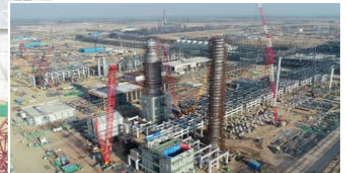
HPCL Rajasthan Refinery Ltd. (HRRL)
