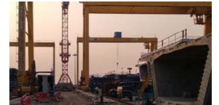
Integrated Anti-Collision System between Tower Crane and Gantry Crane
