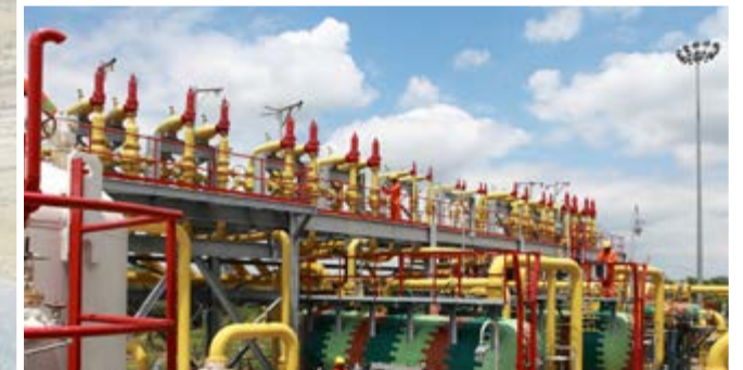
EPC of Gas Processing and Compression Facilities in Rajahmundry
