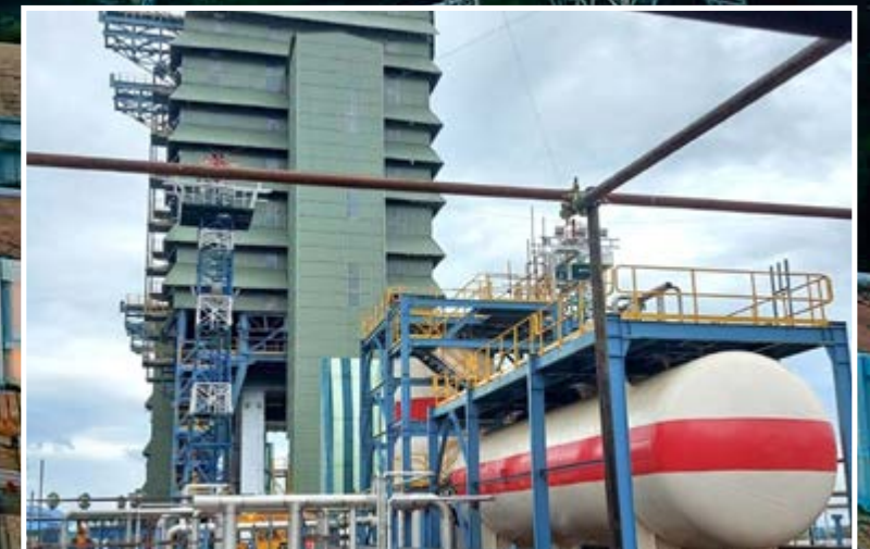
Cryogenic Fuel Storage Facility
