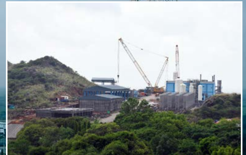
Integrated Cryogenic Engine and Stage Testing Facility
