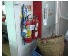
Example of blocking of fire equipment.
