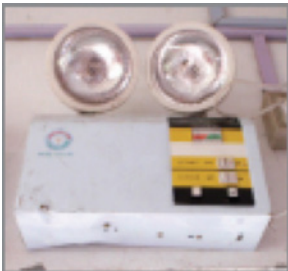
Example of emergency lighting.
