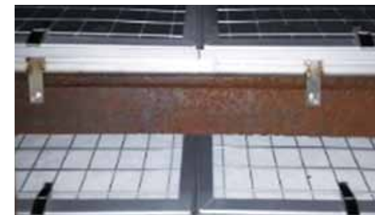
Installed dual filters at deadener booths of the Asan Plant
