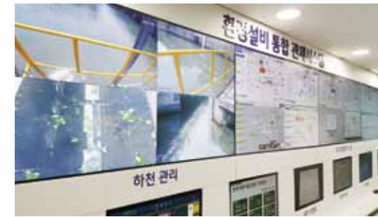
Integrated environmental facility control system at the Ulsan Plant
