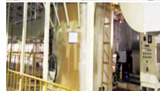
Improved the dust collectors installed at the pre-treatment equipment at paint shops of the Asan Plant
