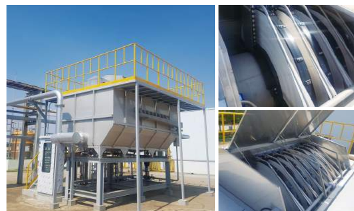
Installation of fiber disc filters at the Asan Plant
