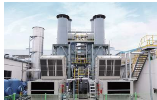
Co-generation facility at the Ulsan Plant
