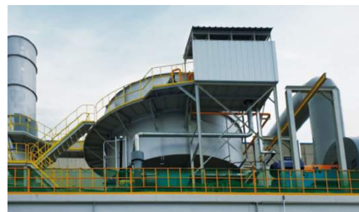
RTO facilities at painting shop 42 line of Ulsan Plant
